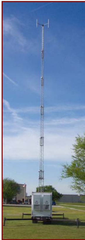
Figure 10. Communication-Site-On-Wheels by Integrated Tower Systems
